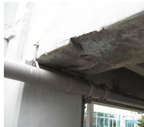
2. Parking structure beam - Before
