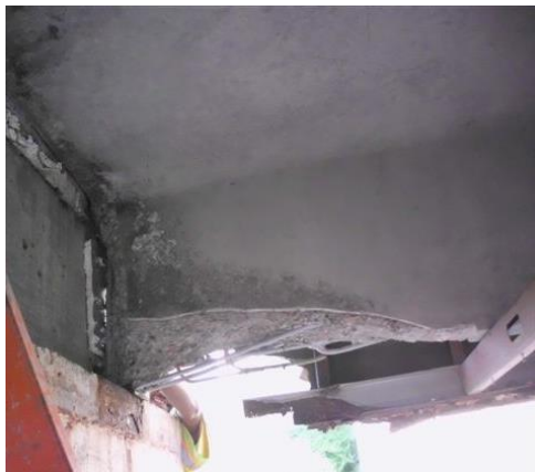
1. Double tee bridge repair - Before
